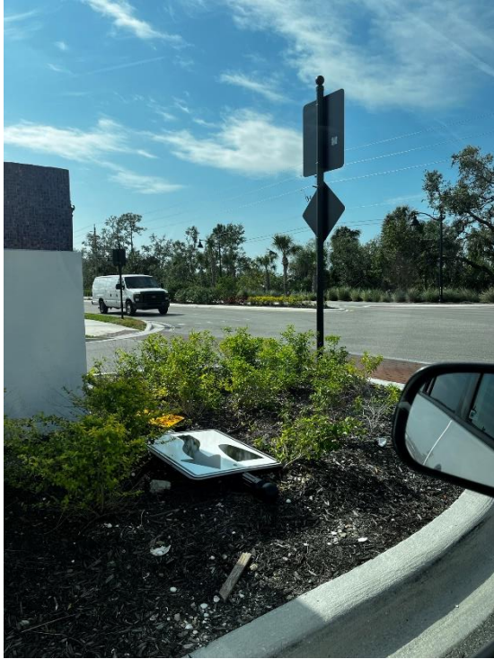
Signs replaced but old sign left on ground
